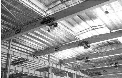
Single girder overhead crane
